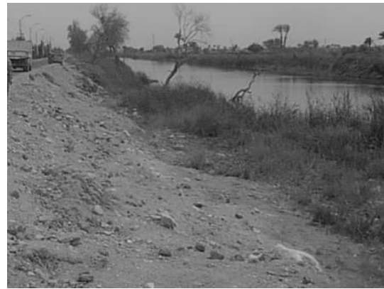
Figure 7 : Slope failure of case 4
