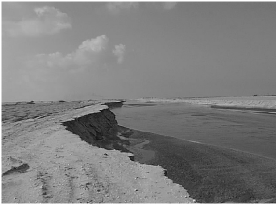
Figure 6 : Slope failure of case 3
