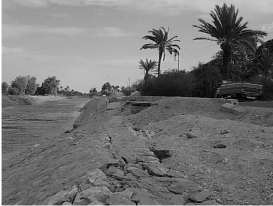
Figure 4 : Slope failure of case 1
